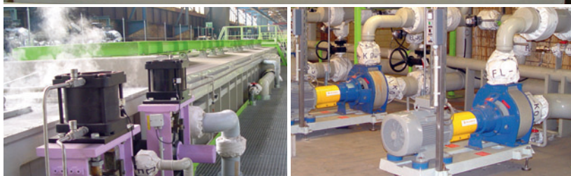
General view of the pickling line and the various tanks
